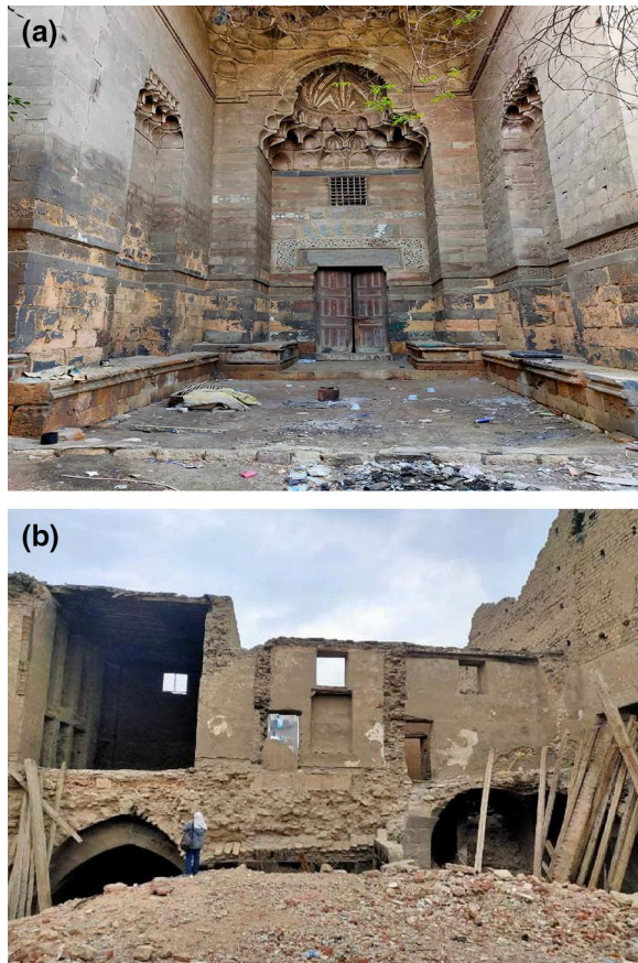
Fig. 3 Soil settlement of the bearing soil underneath the structure of the main entrance and b. The location of the collapsing part of the main façade of the palace due to 1992 earthquake and soil settlement
