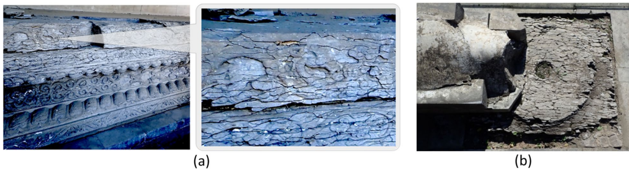
Fig. 2 The layer delamination and laminae deterioration phenomena of tuff monuments in Puyou Temple, Chengde: a base for the Buddhist statues and b pillar stone
