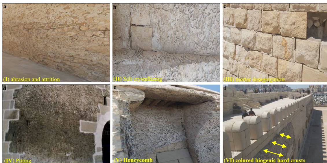
Fig. 2 Shows different deterioration forms affecting Qait Bey Fortress in Alexandria
