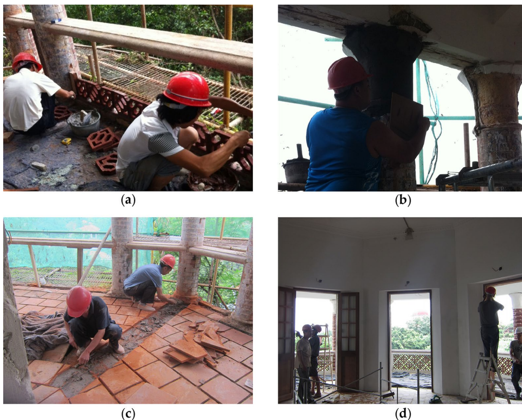
Fig. 4 The restoration project of the former residence of the HSBC bank: a Restoration of the railing at external veranda; b Restoration of the column capital at external veranda; c Restoration of floor of the building; d Restoration of the interior space of the building
