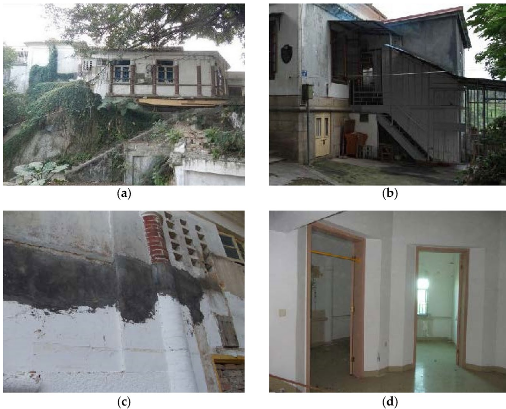
Fig. 3 The damage suffered of the former residence of the HSBC bank: a The external veranda was sealed off artificially; b Additional construction of the building; c The deterioration and damage of walls; d The artificial transformation of the interior space of the building
