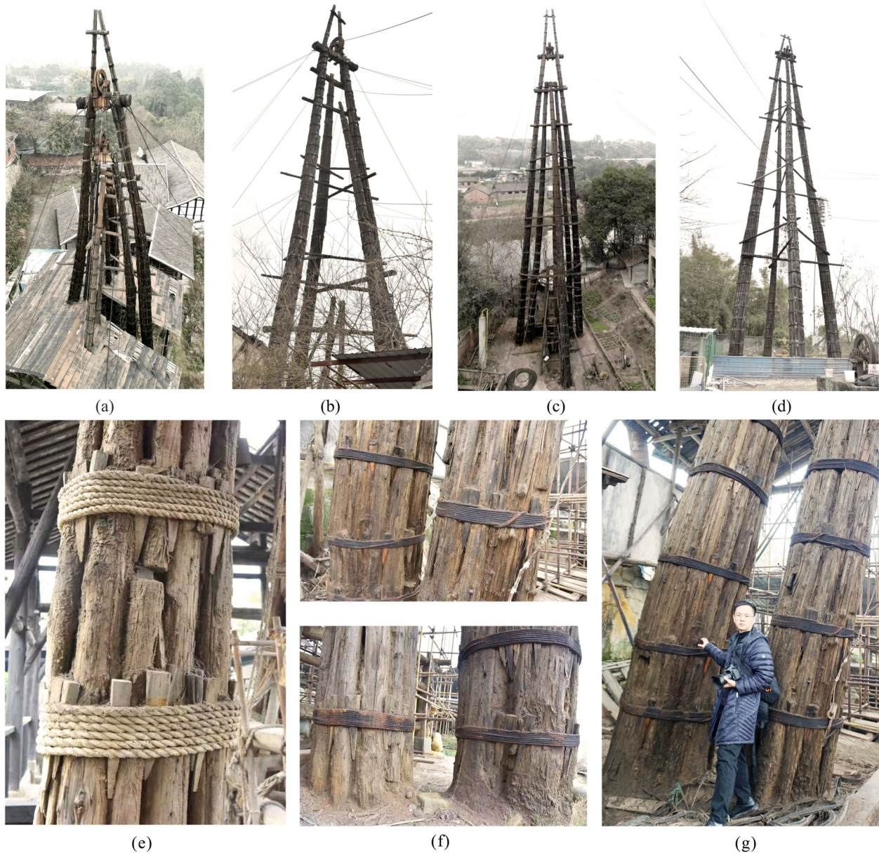
Fig. 3 a–d Existing Tianches in Zigong are generally 20–40 m tall; e–g details of the Tianche columns. Sources: the authors
