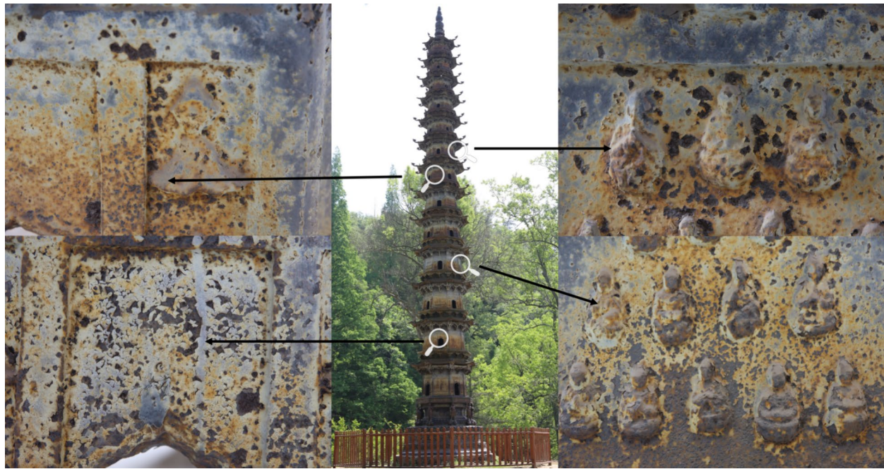
Fig. 1 The corrosion status of the Yuquan Iron Pagoda
