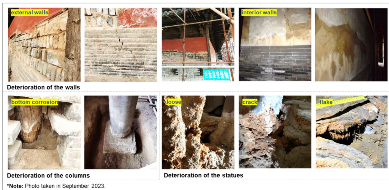
Fig. 2 Deterioration problems of cultural relics in the Great Deliverance Hall
