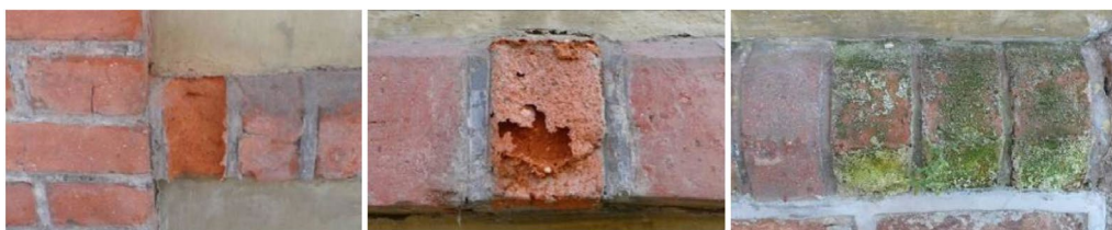
Fig. 14 Corrosion of Attached Building Brick Surface [78]
