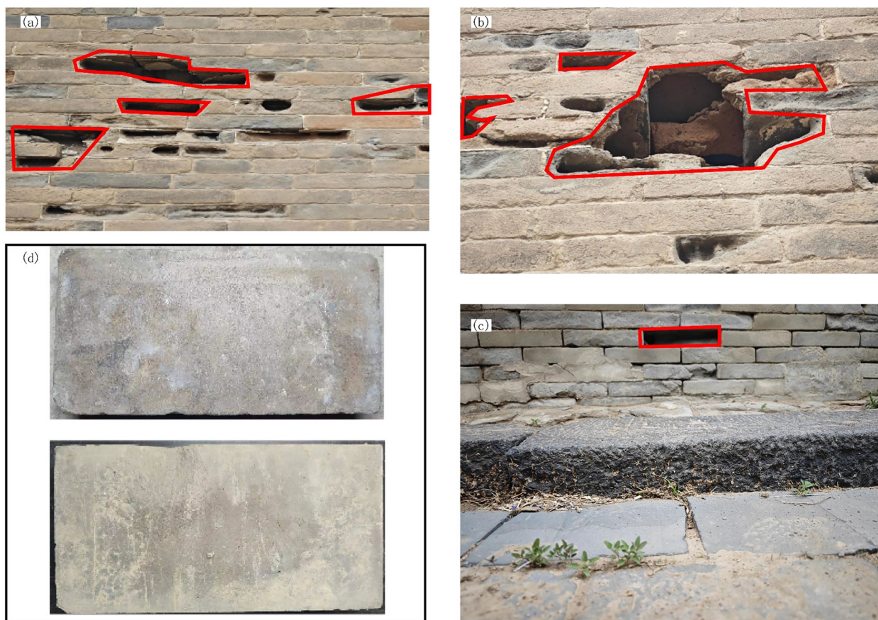
Fig. 13 Material comparison and application of brick repair. (a) The case of discrete severe injury (b) The case of centralized severe damage. (c) Process the replacement area (d) Ancient building brick and archaizing brick
