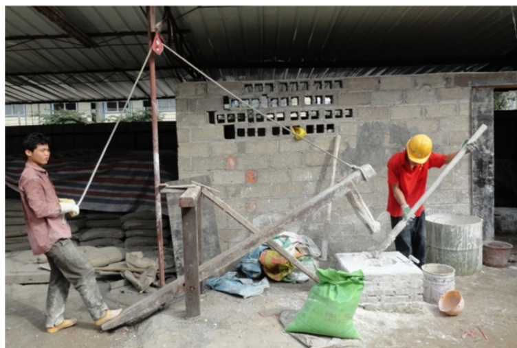
Figure 4 Preparation of lime plaster finishing by tempering for façade restoration in Haikou 2011.
