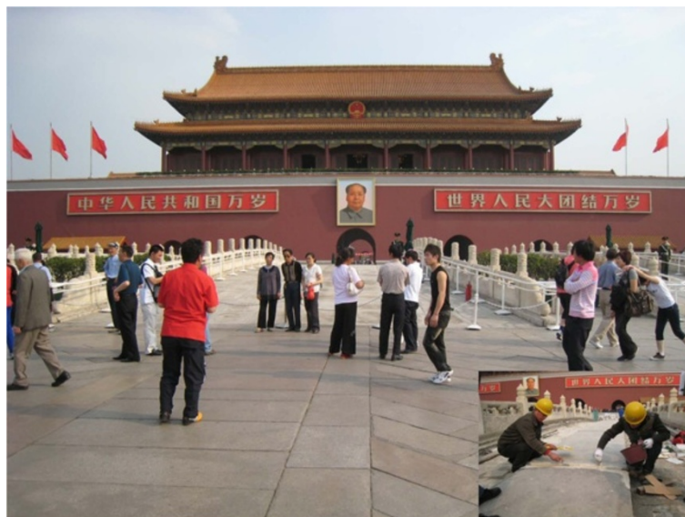
Figure 2 Marble restoration of Golden Bridge in front of Tiananmen Beijing, using NHL2 in 2009 (right) and after restoration (left).
