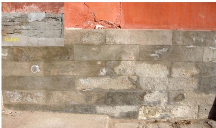
Figure 10 Trail to use lime to restore traditional Chinese green bricks (right after restoration).
