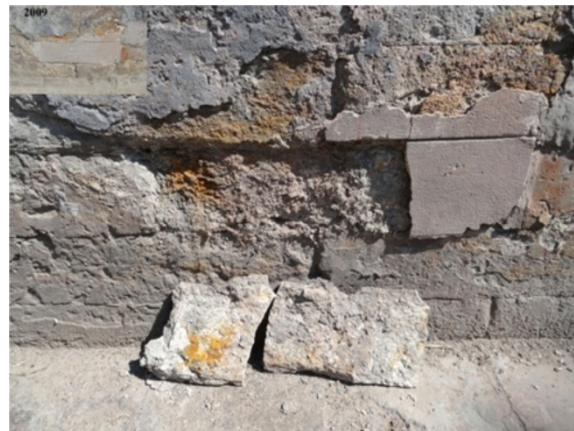
Figure 9 Cement-based mortar applied in 2002 to restore green bricks in Beijing, delaminated in 2012.
