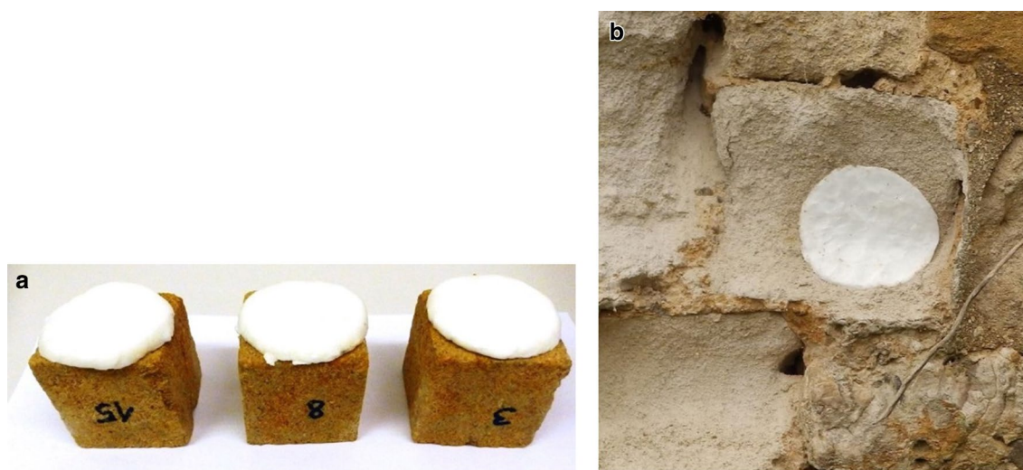
Fig. 2 a Application of poultices on the stone cubes under laboratory conditions; b application of poultices at the boundary wall, Worcester College
