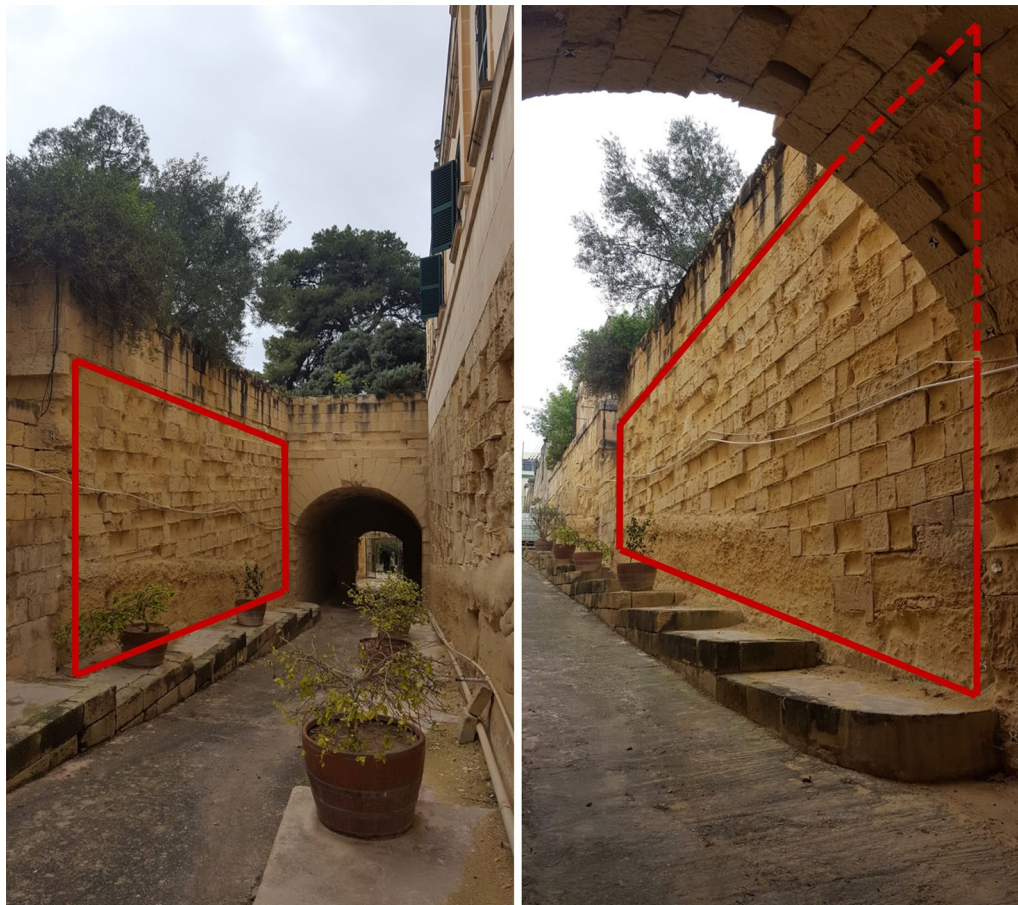
Fig. 1 Retaining garden wall studied in St Philip's Garden, Floriana, Malta. (Left: top view; Right: bottom view)
