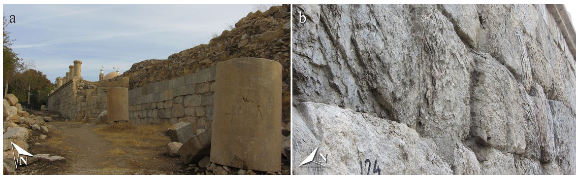
Fig. 11 a Images of the mass of soil behind the western wall of the monument; b close-up image of deteriorated blocks on the wall in the northwest area of the monument
