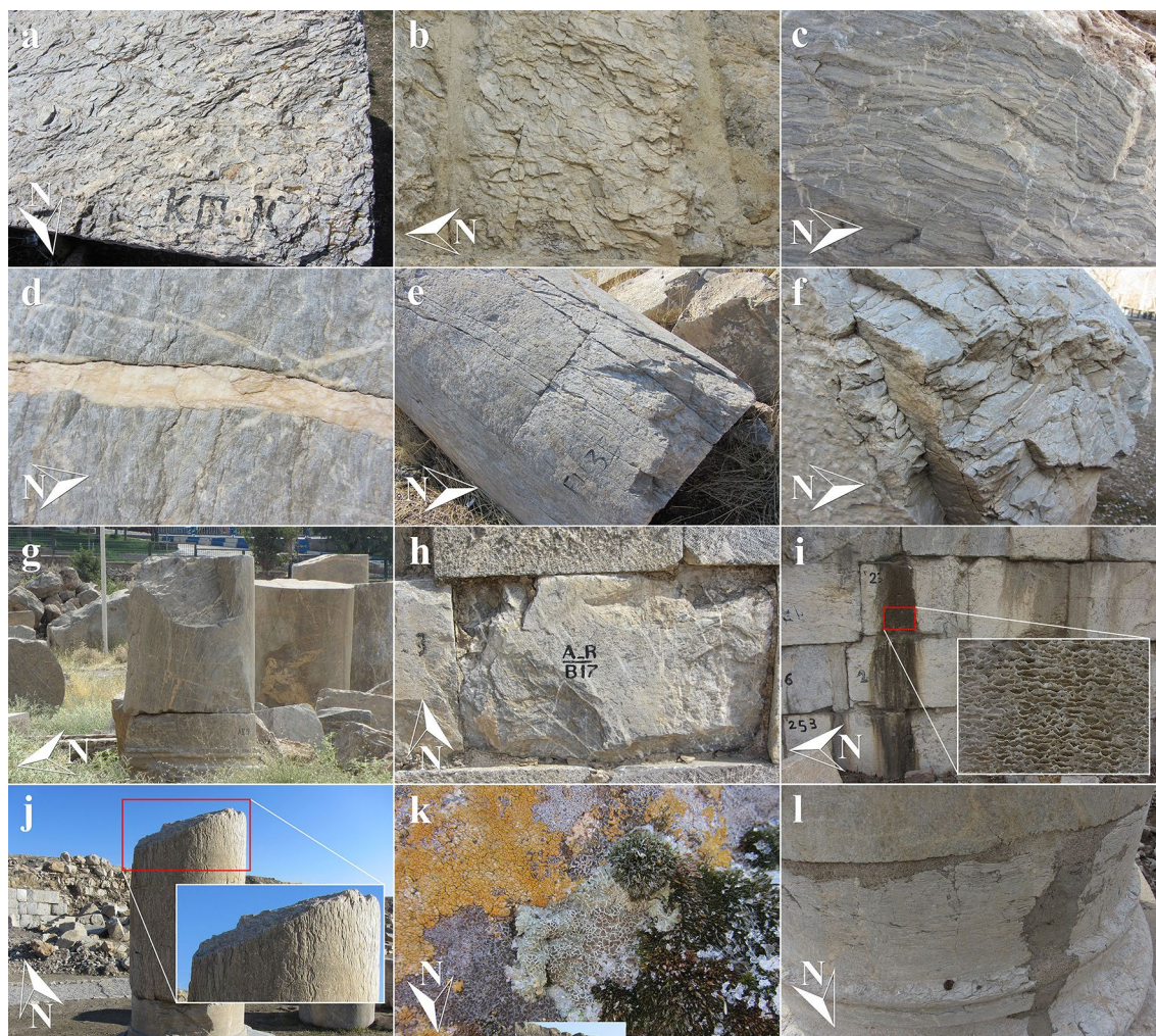
Fig. 6 Image of decay patterns of the stones used in the construction of Anahita Temple of Kangavar. a The scaling occurred in the south side of the monument which located in the area around the main building; b the scaling of the stone blocks forming the wall of the western side; c delamination of the layers of stone, the southern side of the monument; d the image showing the detachment of two layers with different colours from the columns located on the south side of the monument; e cracking occurred in a stone column, the eastern side of the site; f the detachment in a stone column on the western side of the monument; g the image of the bursting and the loss of stone in the south side of the monument; h bursting of the edges in the blocks of wall construction on the south side of the monument; i Alveolization and the formation of hard depositions on the surface of the wall of the western side of the monument; j the occurrence of the rillenkarren phenomenon in one of the columns located on the southern side of the site; k the growth of lichens on the stone surface located on the eastern side of the monument; l unsuitable intervention in the form of widespread use of cement to fill the loss parts of stones; the image shows the columns located on the western side of the monument
