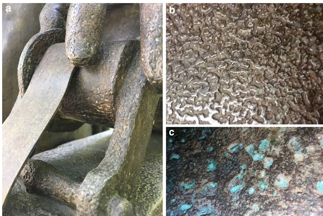
Fig. 2 Condition issues observed on the Morse sculpture (I). Photographs showing (a) a detail of sculptural surface loss, (b) typical pitting and loss pattern on exposed surfaces, and (c) a detail of active corrosion present in the recessed areas
