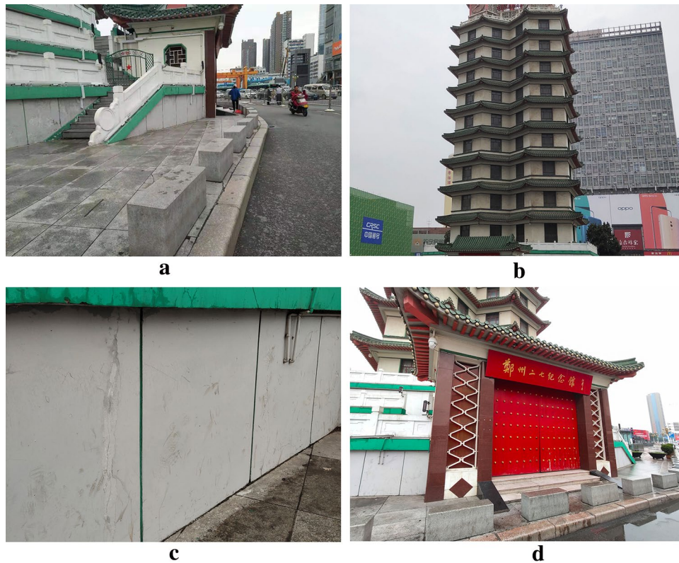
Fig. 7 Damage to different parts: a outdoor floor; b main structure; c non-structural components; d door
